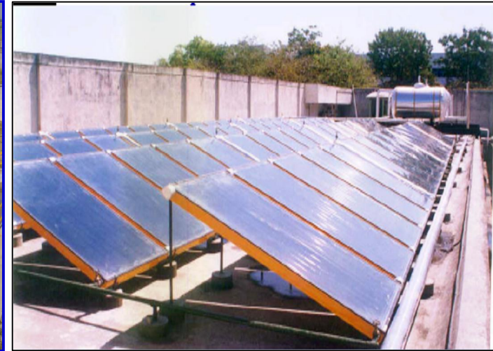
Solar Water Heating for Canteen
